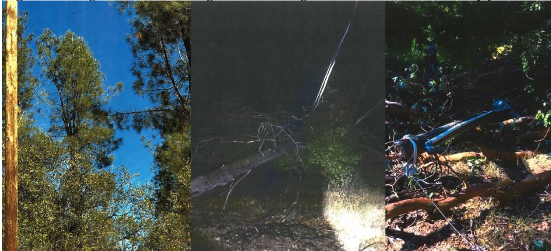
Figure 8: (left) Sac Valley Veg Related Damage – Tree branch resting on conductor Figure 9: (middle) North Coast Veg Related Damage – Tree fell into secondary line Figure 10: (right) North Coast Veg Related Damage – Tree took down secondary pole
