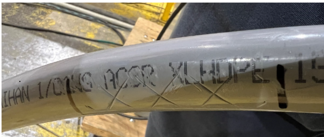
Figure 6-15: Sample 3.2.2 - 35 kV, 1/0 AWG ACSR Condition after Test
