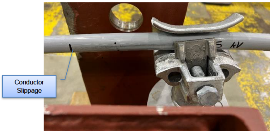
Figure 6-10: K-Line KL46SK - Typical 1/0 AWG ACSR (35 kV) Conductor Condition after Slip Test
