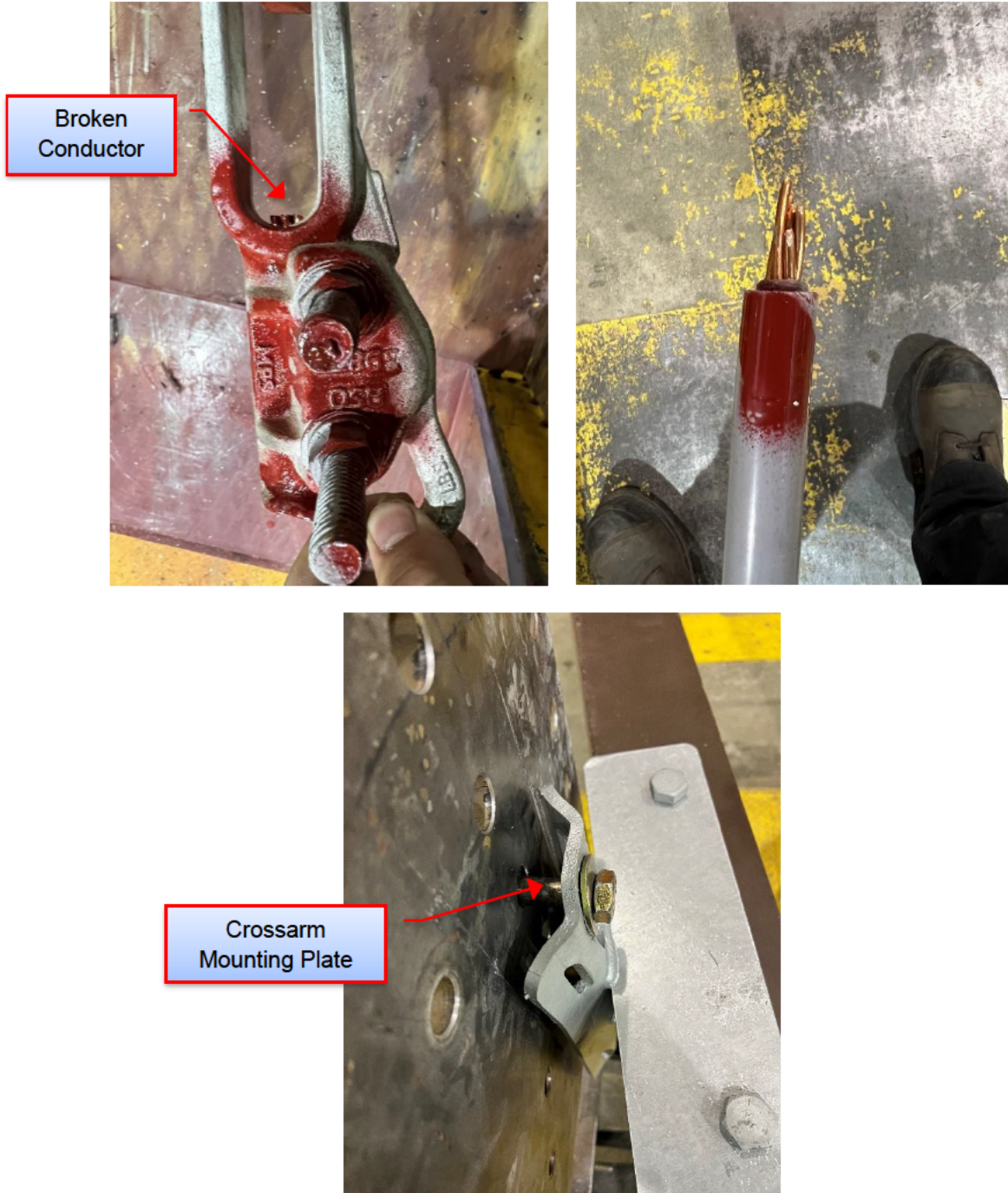
Figure 6-8: Sample 1.1 – Failure Location
