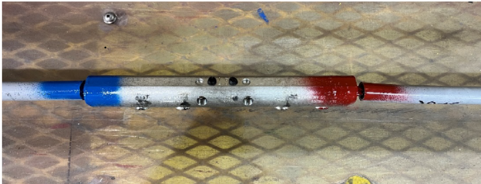
Figure 3-5: Sicame MTRS-01 Installed on 15 kV 1/0 AWG, 6/1 ACSR
