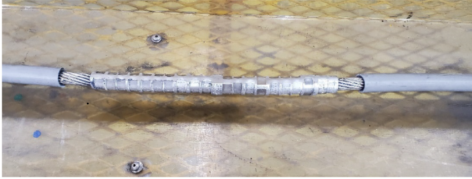
Figure 3-4: Hypsplice™ YDS311AT Installed on 22 kV 397.5 kcmil, 19 strands AAC
