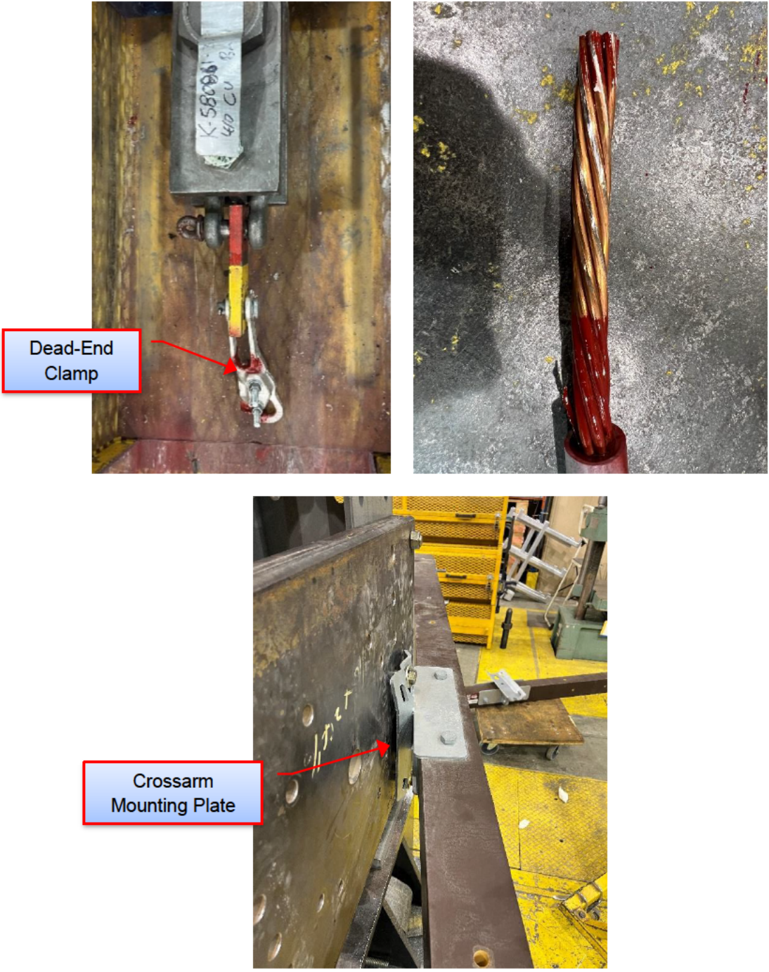
Figure 6-16: Sample 3.3 – Failure Location
