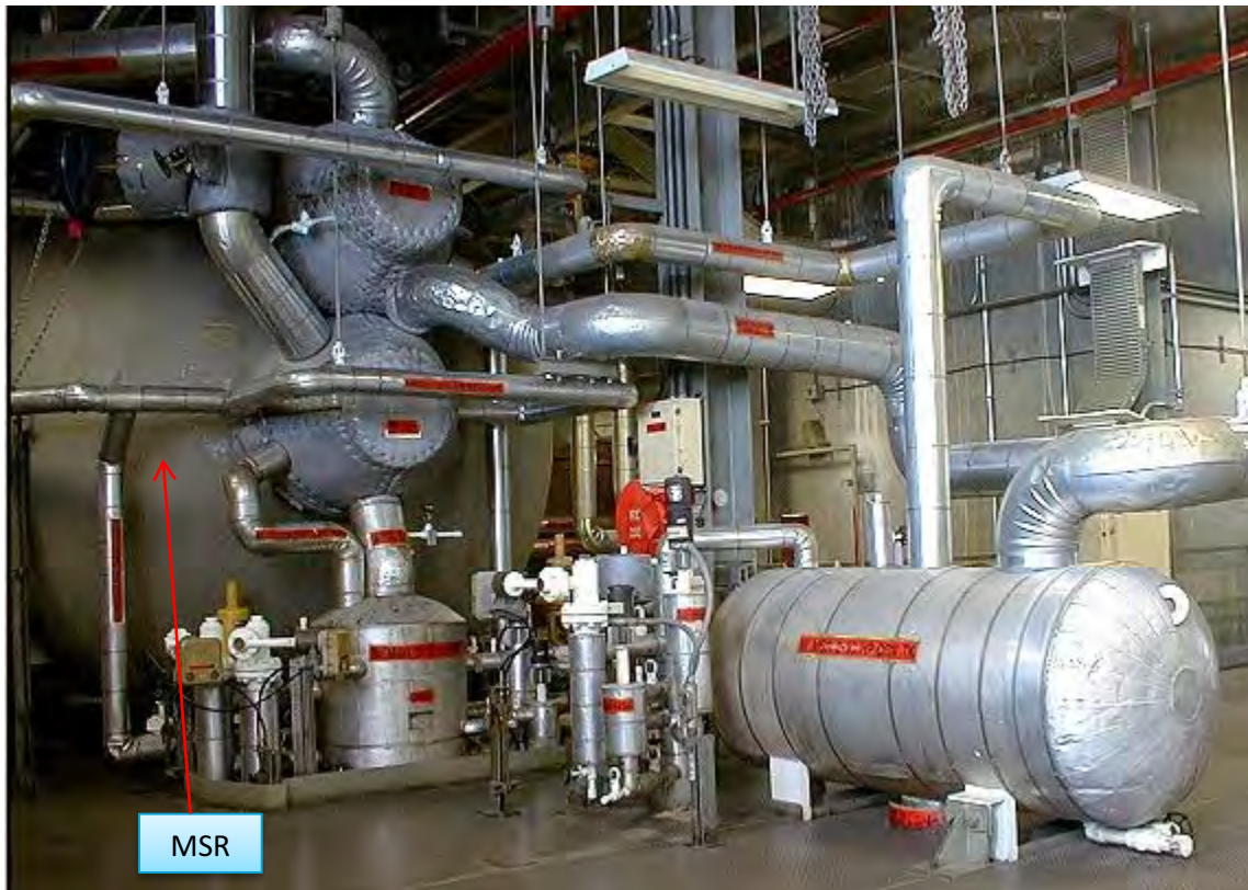
Moisture Separator Reheater (left center of photo)
