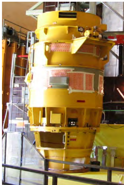
Reactor Coolant Pump motor
