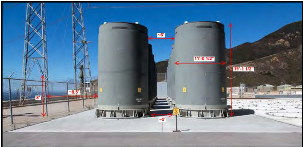
Figure 4-25: Elevation View of Canisters on New Pad
