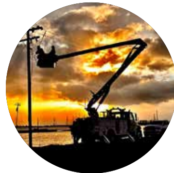
Alvah Group, Inc.: Distribution poles
