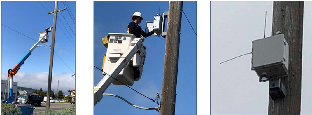
Figure 3. DRLM Sensor Installation
