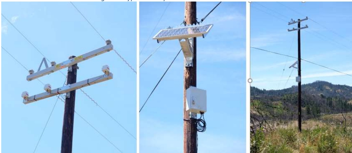
Figure 9. Typical solar-powered RF data collection unit
