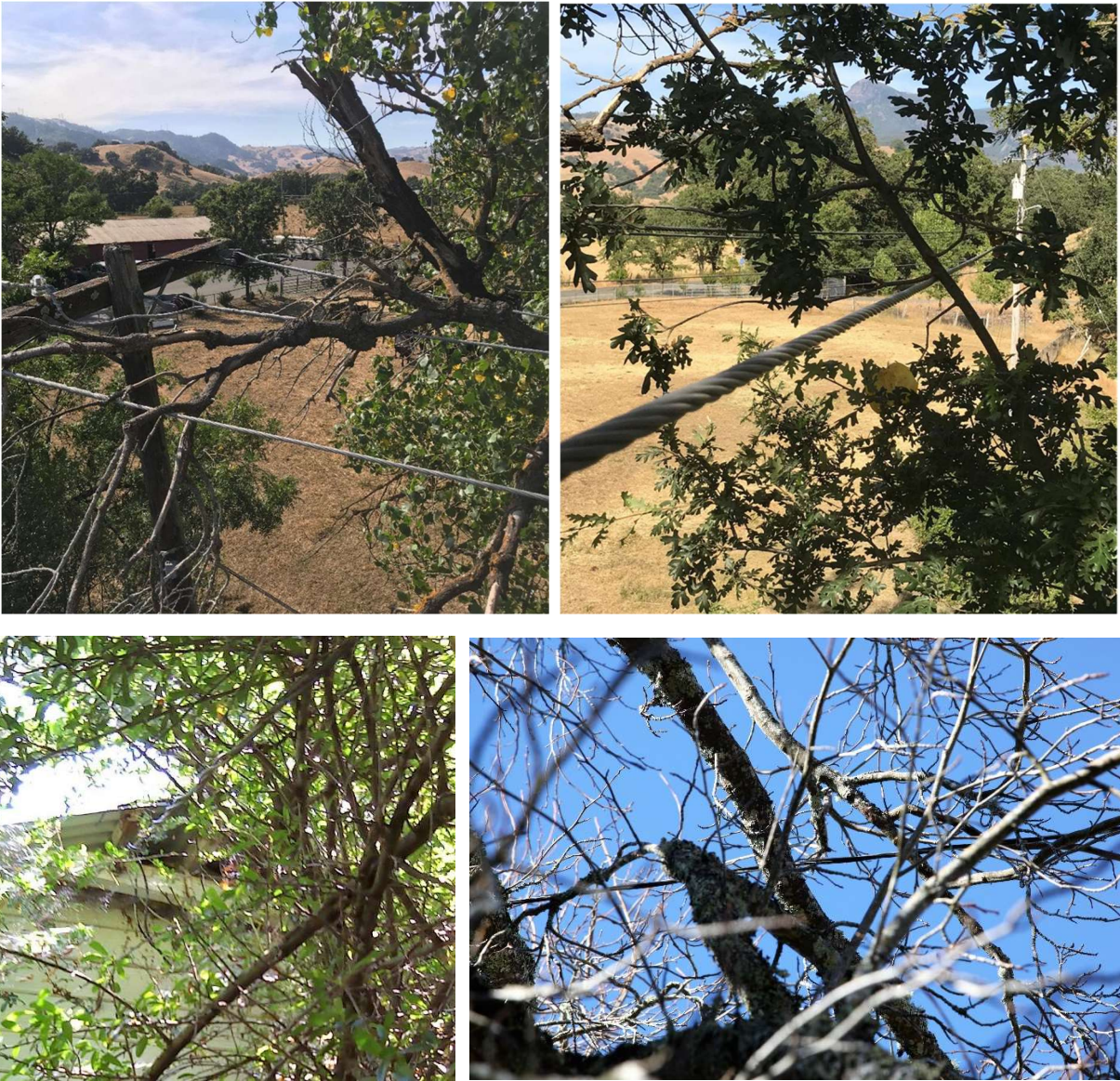
Figure 11. Examples of vegetation on secondary conductors
