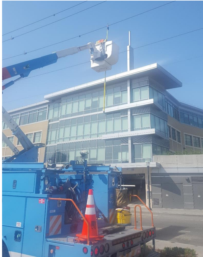
Figure 5: Phase Identification Tracker Usually Used by PG&E Line-Crew Staff
