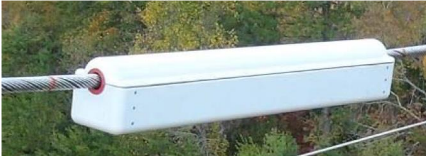
Figure 3-1 DSR on a Transmission Line
