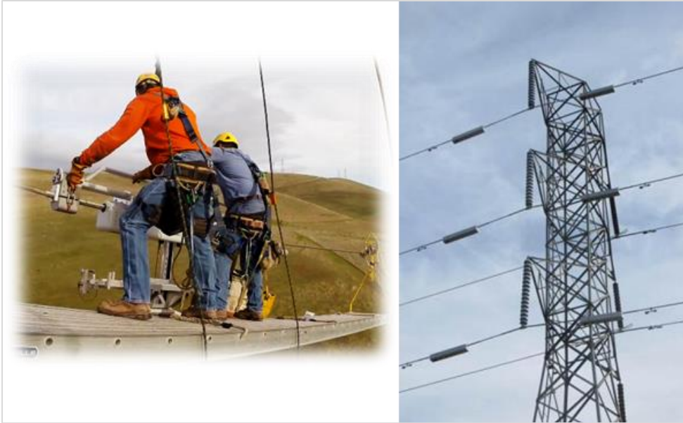
Figure 4-1 Tower on Las Positas-Newark 230 kV line with 6 units installed and Crew Installing Unit
