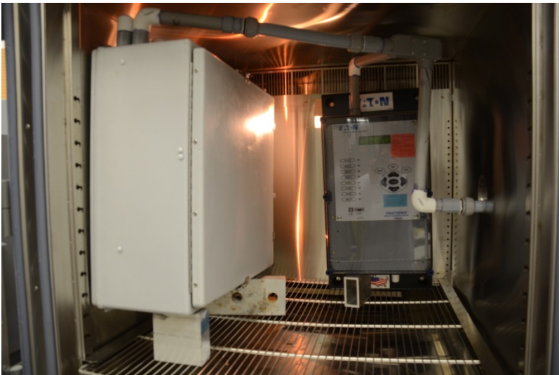
Figure 4-2 SCADA Equipment Test Set Up
