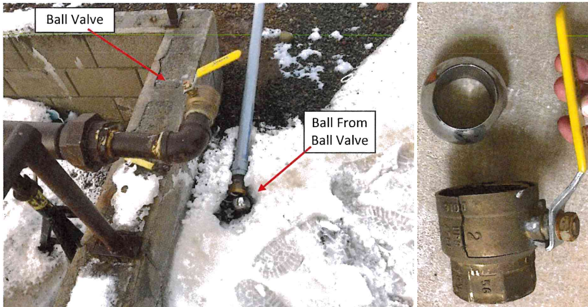
Figure 2. Ball Valve with Broken Ball and Disconnected Piping
