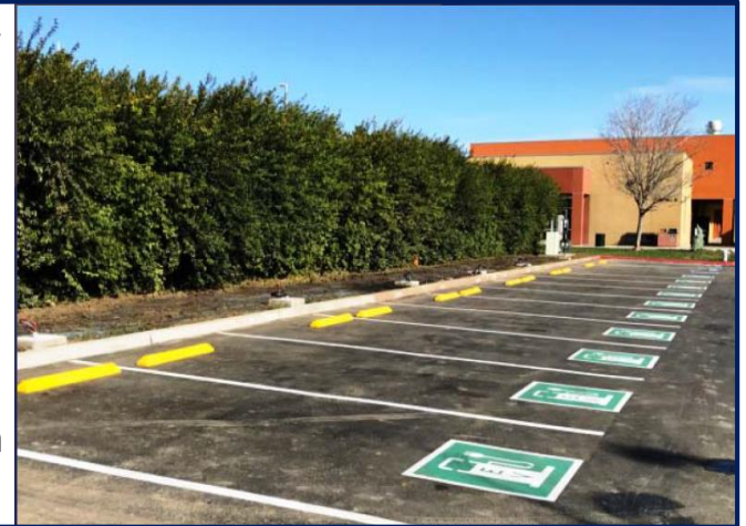
Completed striping and preparation for EV charger installation at first site, Merced Community College, Los Banos
