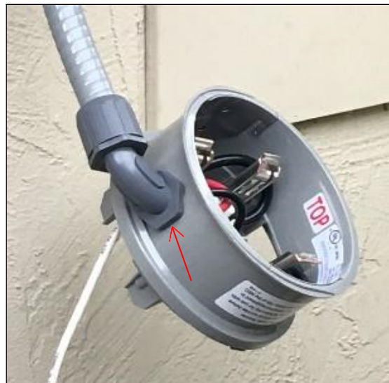
Figure 7. Point of Interconnection
