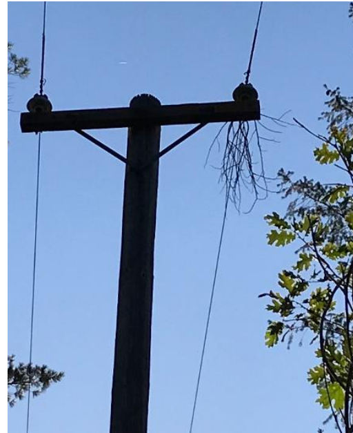
Figure 2 – Vegetation Debris Near 98 Gamble Rd, Oroville
