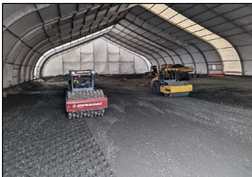
Clean imported backfill is placed in the excavations and compacted to the final grade.
