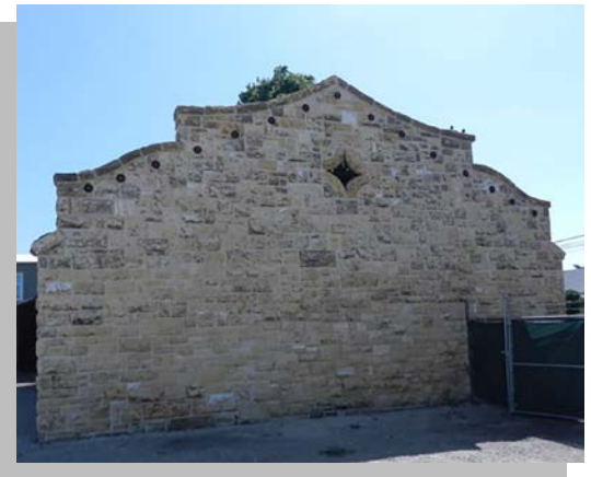
PG&E retrofitted the historic gas building, shown above, which will remain on-site.
