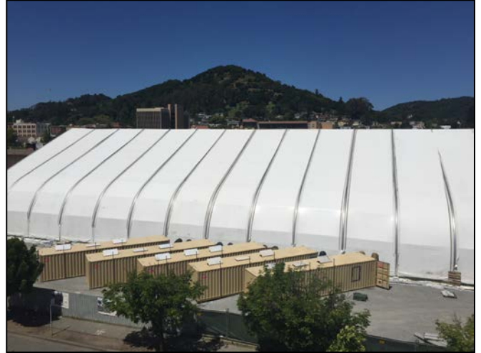
Most work will be conducted within a tent, similar to the one shown above, to control dust and odors.
