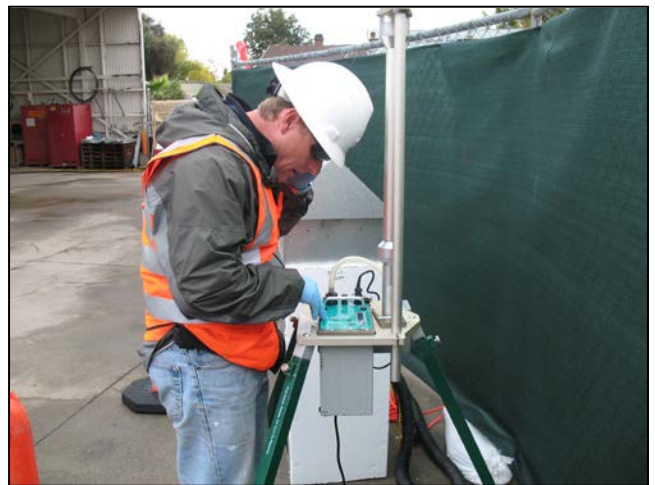
PG&E uses air monitors, like the one shown above, to assist in keeping air quality within levels established by DTSC to be protective of public health.
