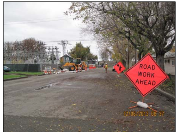
From January 7 to 9, 2013, the portion of 1 st Street between Main and Market Streets (as shown above) will be closed to through traffic and pedestrians while PG&E conducts remediation work.
