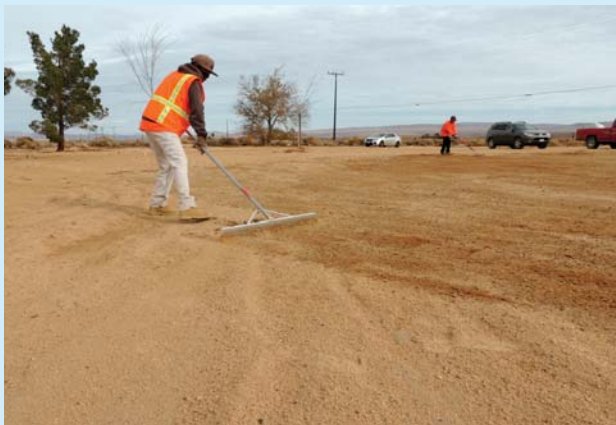
Dakota Nowlin, current Workforce Development participant, prepares a property for restoration and re-planting.
