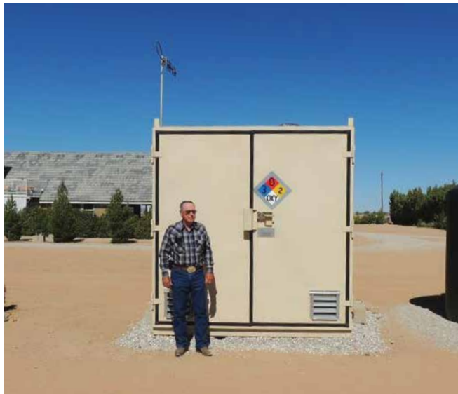
Joe Summers next to his new Whole House Replacement Water Treatment System
