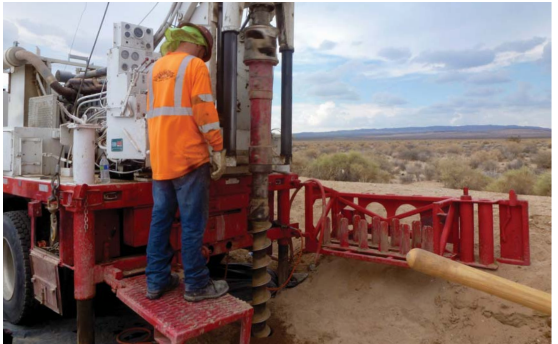
Last year, crews installed additional groundwater monitoring wells as part of the Updated Chromium 6 Background Study.
