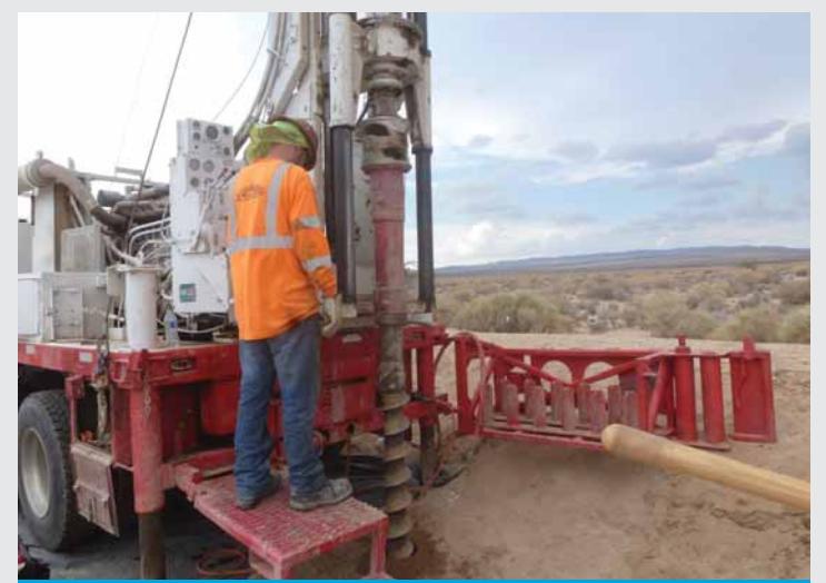
Crews will install additional groundwater monitoring wells as part of the updated chromium 6 background study.
