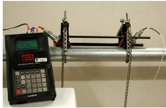
Figure 1: Flow meter installed in the field.
