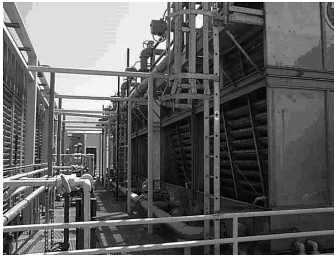
Figure 5.01: Cooling Towers from a Chilled Water Cooling Plant (Source: Integral Group)
