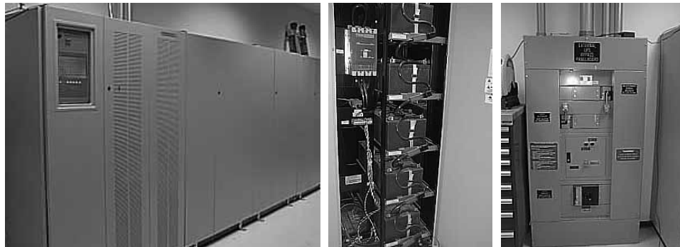
Figure 10.01: Typical UPS units (Source: Integral Group)
