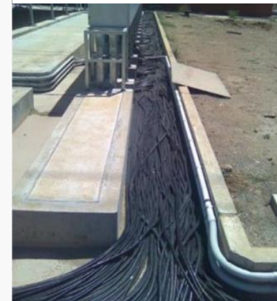
Hard wired substation
