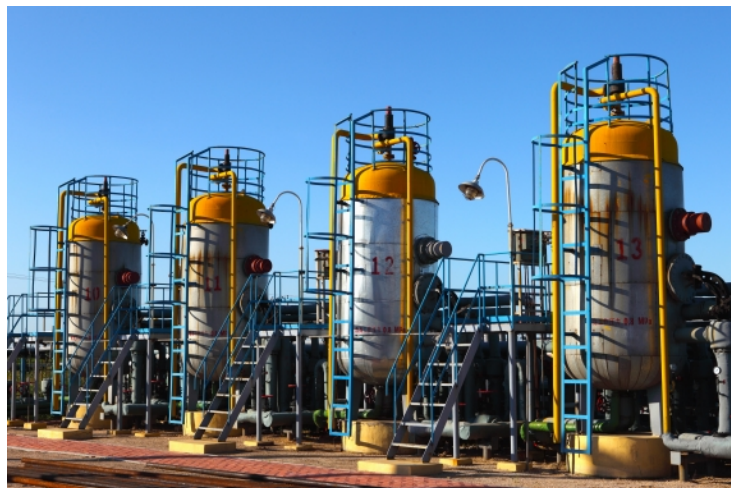
Figure 7 Industrial Pressure Swing Adsorption Plant (AIChE, 2014)
