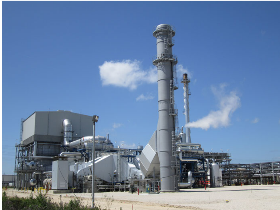
Steam reforming unit open in 2012 by Air Liquide in La Porte (TX)
