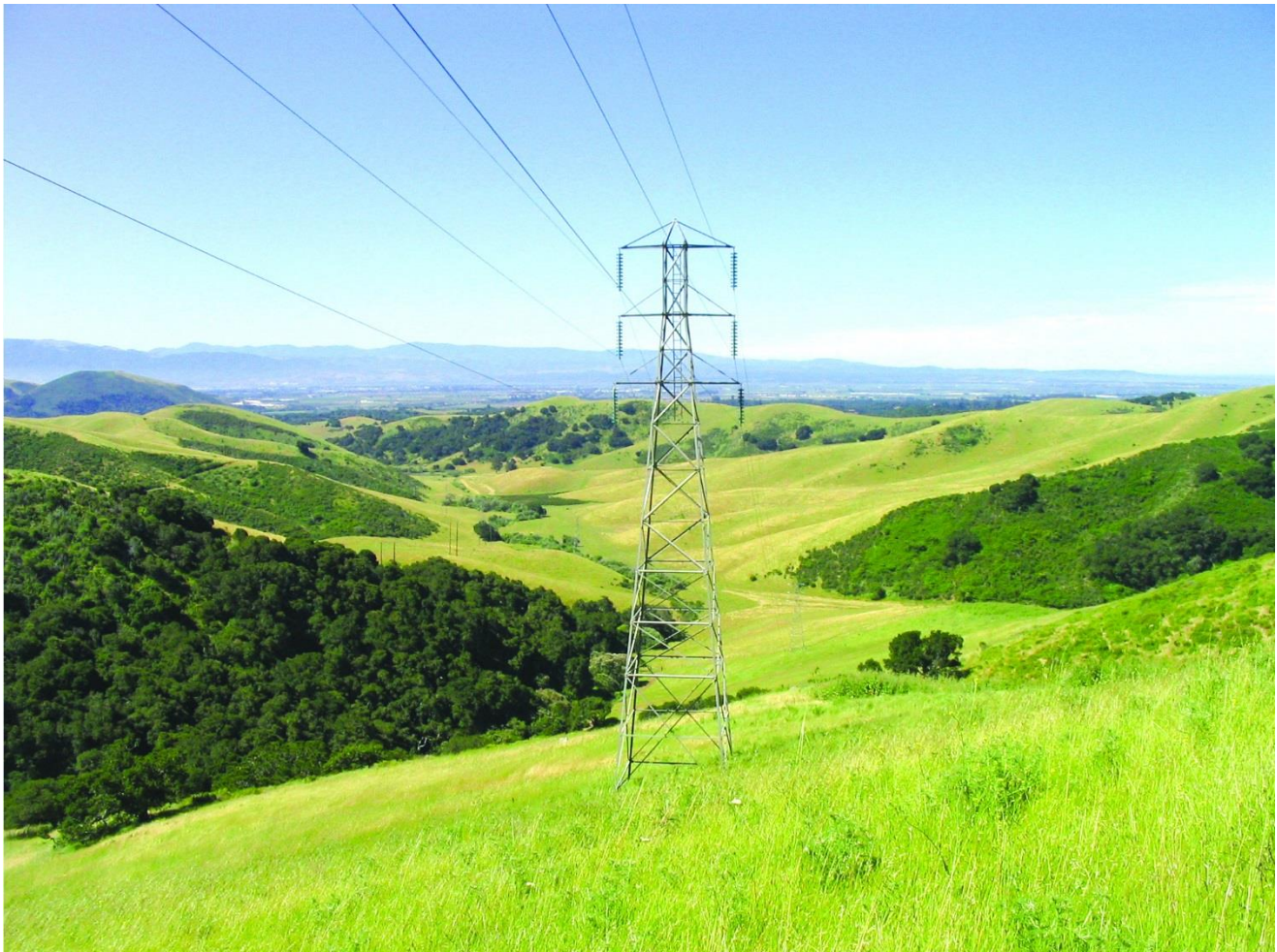
Figure E-2. Electric Transmission Facilities With Steel Structure
