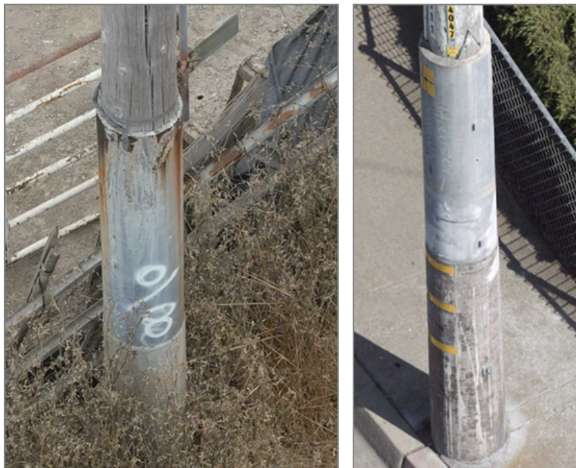
Figure 17. Wood Pole with Steel and Concrete Casing
