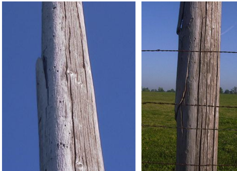
Figure 2. Poles with Compression Wood
