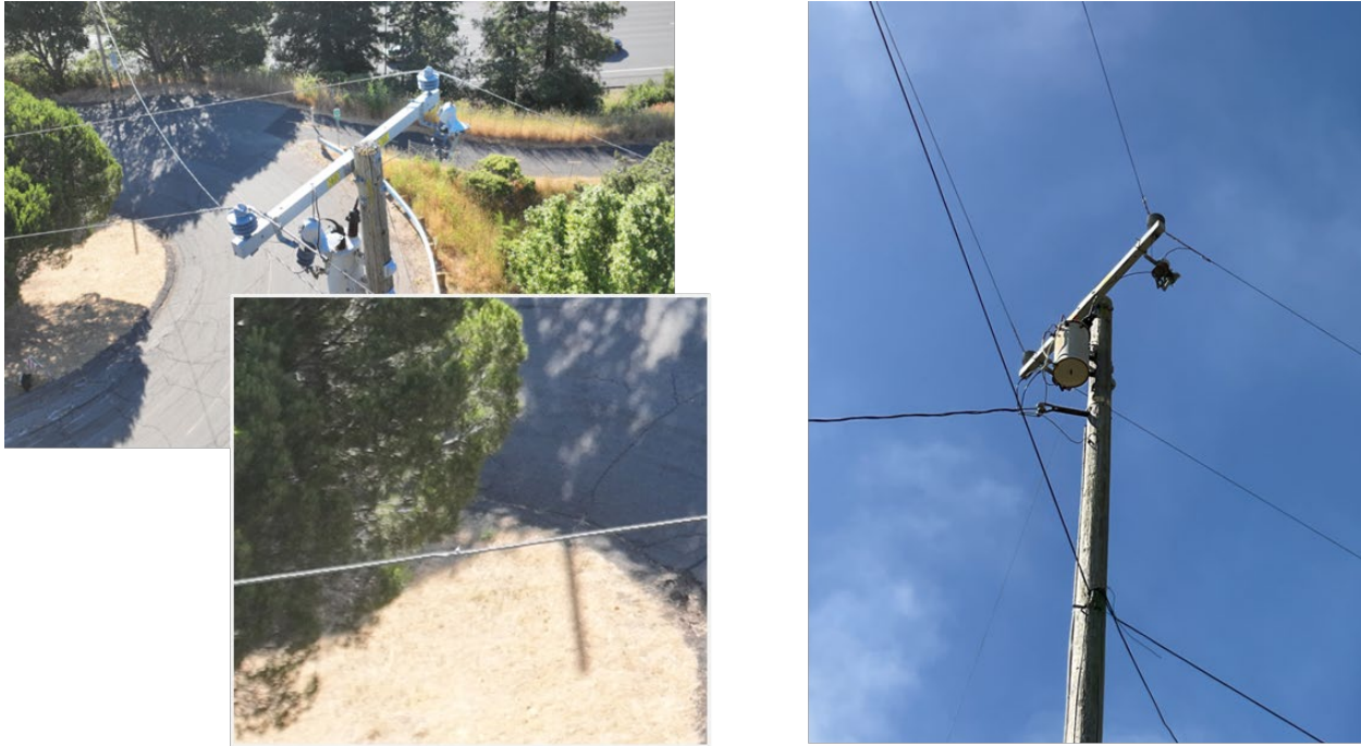
FIGURE PG&E-8.3.8.3-1: IMAGES OF AERIAL CONDITIONS IDENTIFIED (1 of 3)
