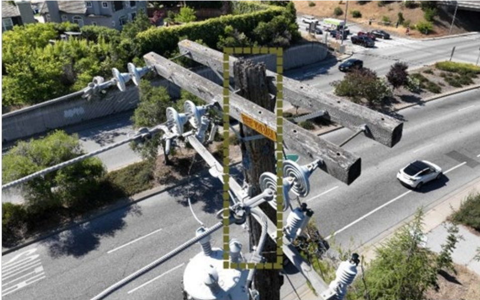
FIGURE PG&E-8.3.8.3-3: IMAGES OF AERIAL CONDITIONS IDENTIFIED (3 of 3)
