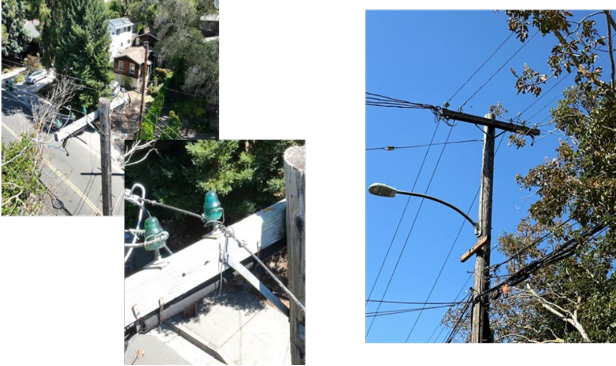
FIGURE PG&E-8.3.8.3-2: IMAGES OF AERIAL CONDITIONS IDENTIFIED (2 of 3)
