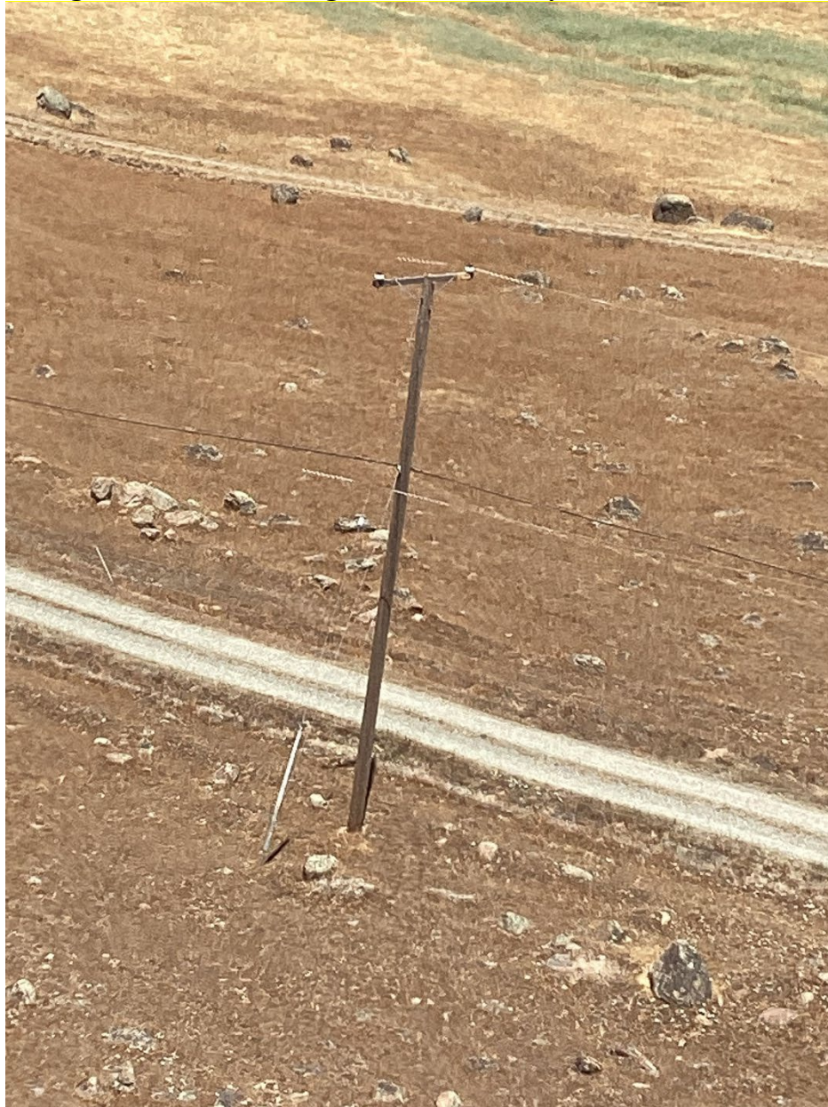
Figure 19: Wind Damage in Sutter County – Broken Tie Wire
