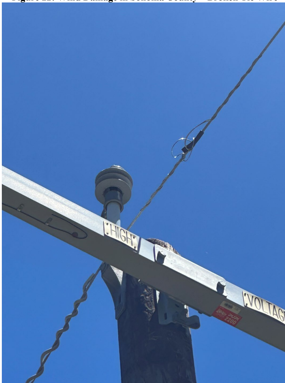
Figure 22: Wind Damage in Sonoma County – Broken Tie Wire
