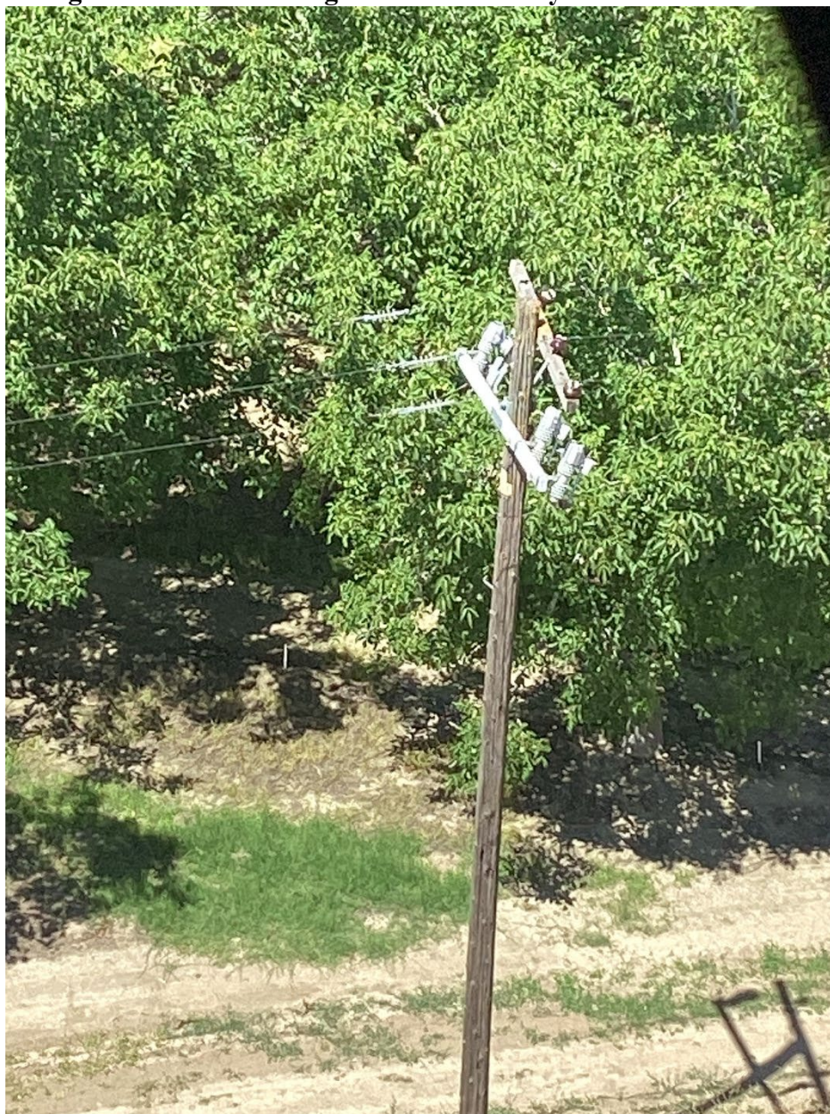
Figure 20: Wind Damage in Sutter County – Broken Insulator
