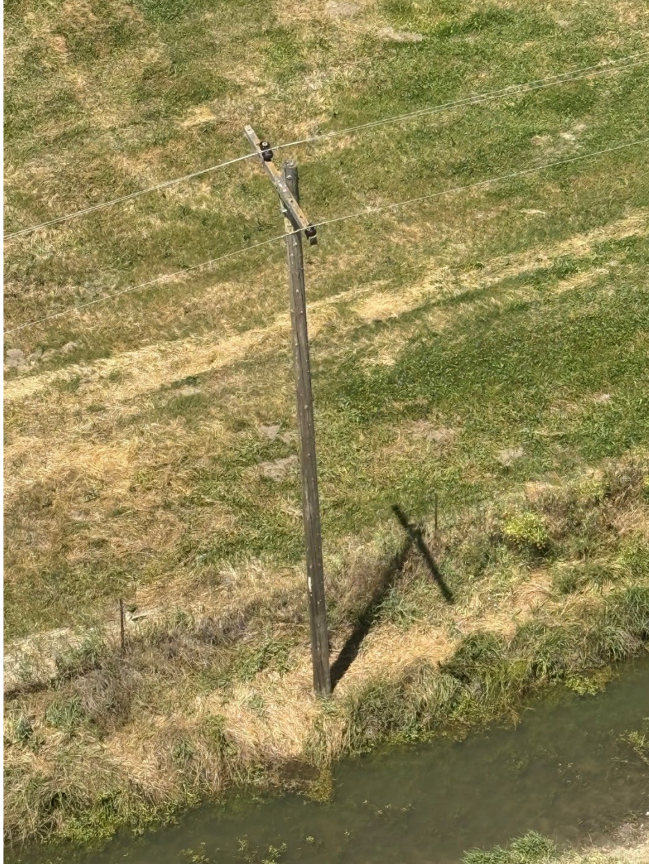
Figure 21: Wind Related Damage in Glenn County – Broken insulator
