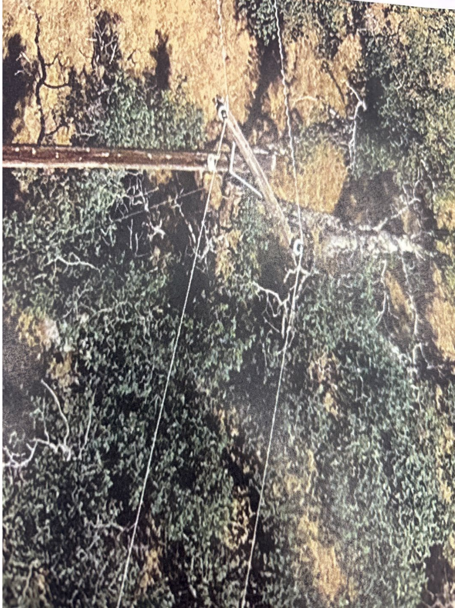
Figure 20: Wind Related Damage in Colusa County – Broken crossarm
