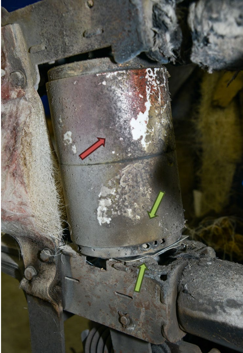
Figure 16. A-phase vacuum bottle detached from the top insulator. Evidence of arcing to the bottom metallic cap and connecting arm (green arrows). Clean burn pattern on the front-facing side (red arrow).
