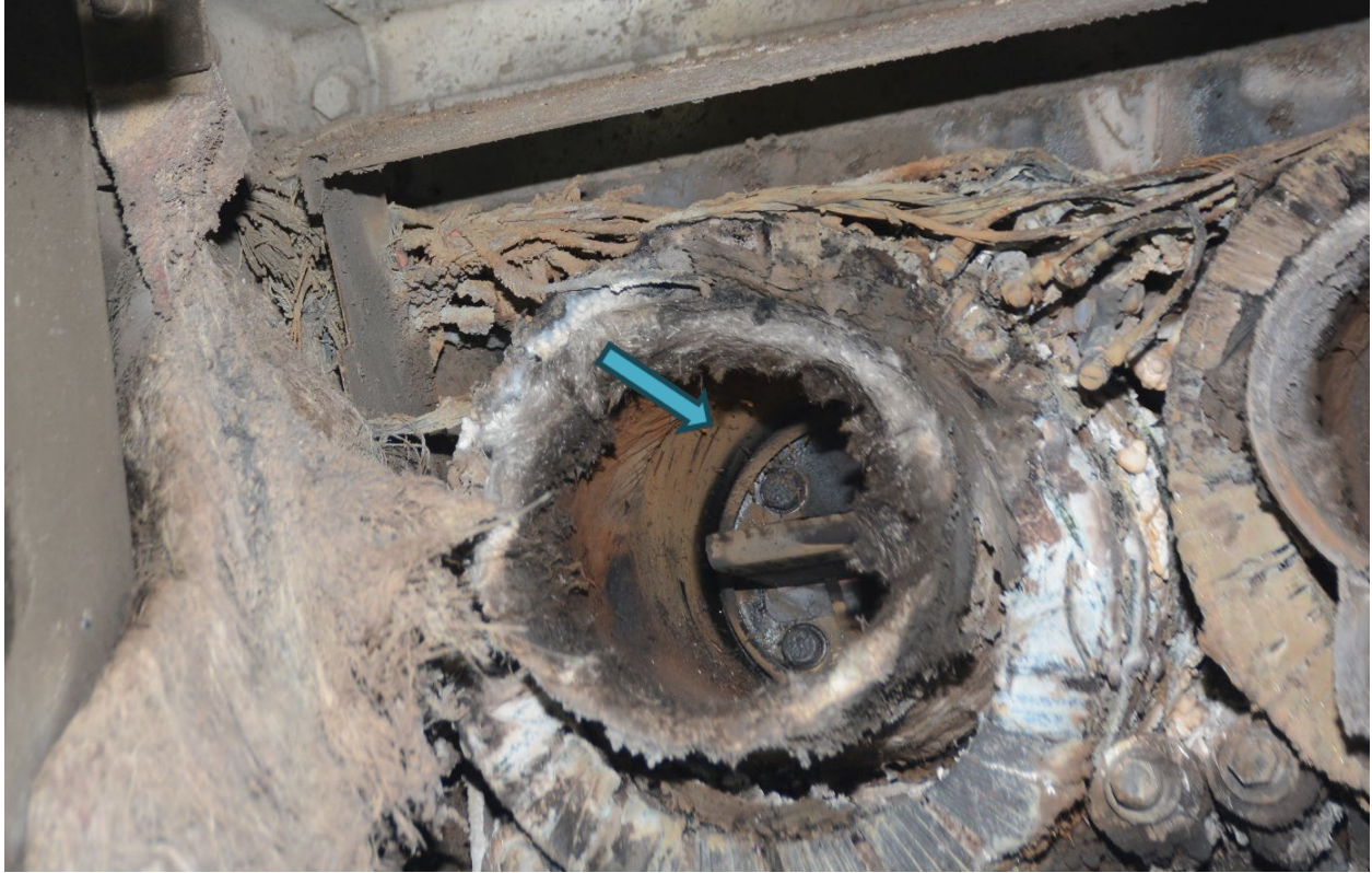
Figure 24. Back, top, A-phase side of Cell No. 5 with most severe damage. No evidence of arcing on bus work connections (blue arrow).
