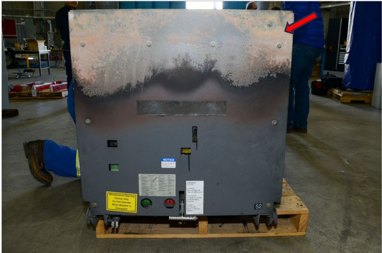
Figure 13. Discoloration and clean burn patterns on the top third of the front face on Incident Breaker No. 52 (red arrow).
