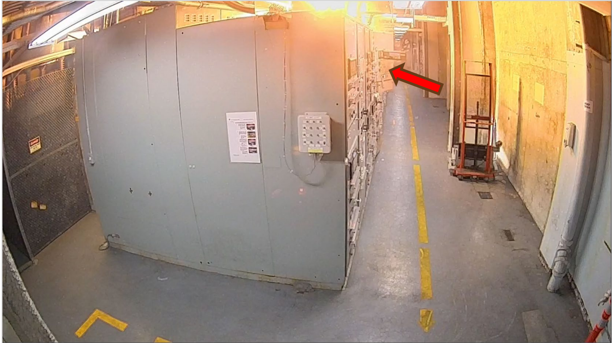
Figure 4. Ignition following arc-flash event in Cell No. 5 (red arrow).
