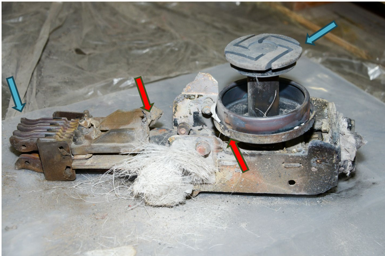
Figure 17. Detached top B-phase connecting arm showing evidence of arcing on the arm and metallic cap of the vacuum bottle (red arrows). No evidence of arcing on connecting teeth or vacuum bottle contacts (blue arrows).
