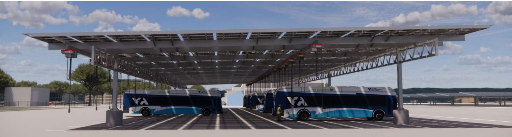
Figure 1: Electric buses charging beneath a solar canopy at VTA's Cerone Yard.
