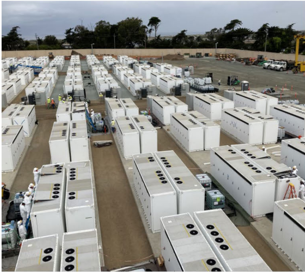
Megapack aerial view looking west
