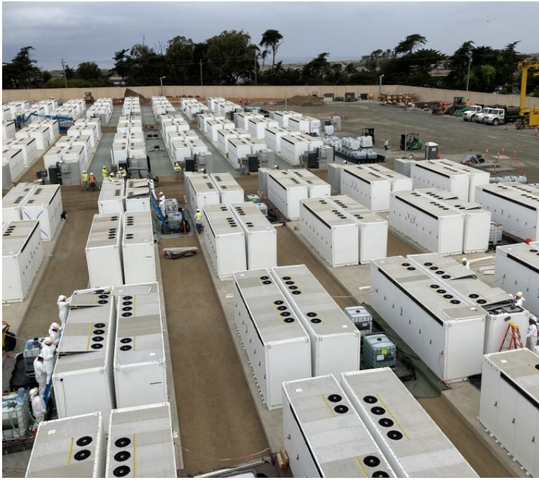
Megapack aerial view looking west
