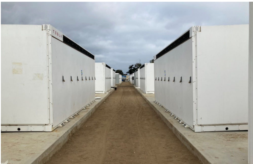
Example Megapack lane looking west
