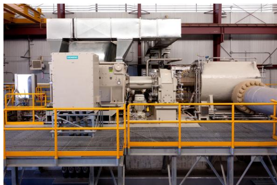
Figure 18 – Delevan K-1 Compressor Unit
