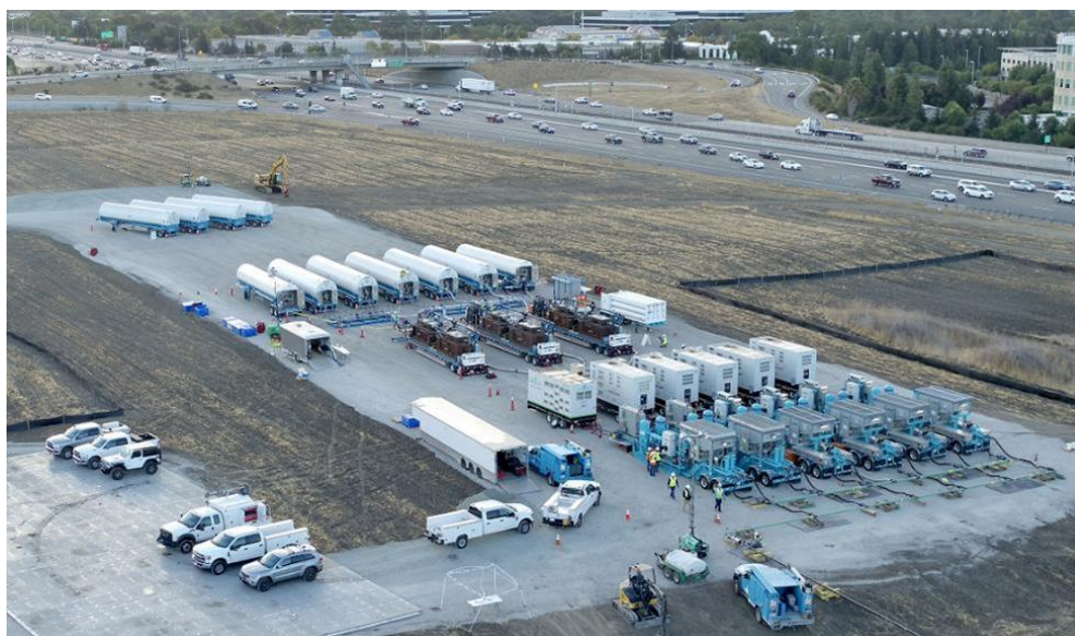
Figure 24 – A Large-Scale LNG Injection Site in Dublin, CA Supporting a Planned Gas Outage
