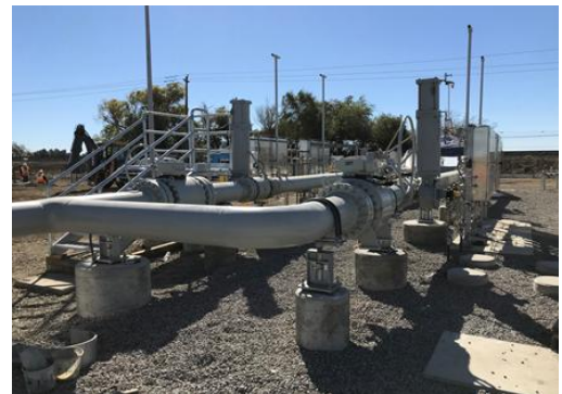
Figure 20 – M&C Complex Station-Above Ground
