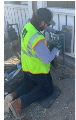
Figure 22 – PG&E Employee Working on Customer Connected Equipment
