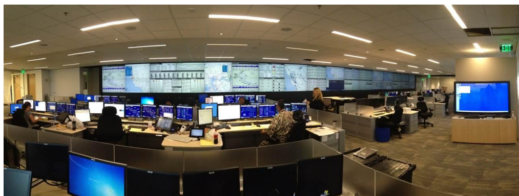
Figure 55 – PG&E’s Gas Control Center Features a 90 Foot-Long Video Wall with Current Operational Information to Augment the Gas SCADA System
