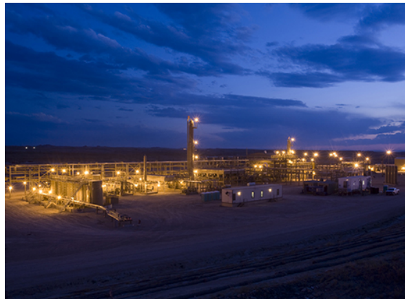
Figure 1 UOP Russell modular cryogenic plant
