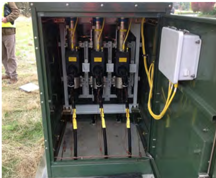
Figure 6 PMI-4R Single Phase Vacuum Fault Interrupter - Source Side (replacement construction shown)
