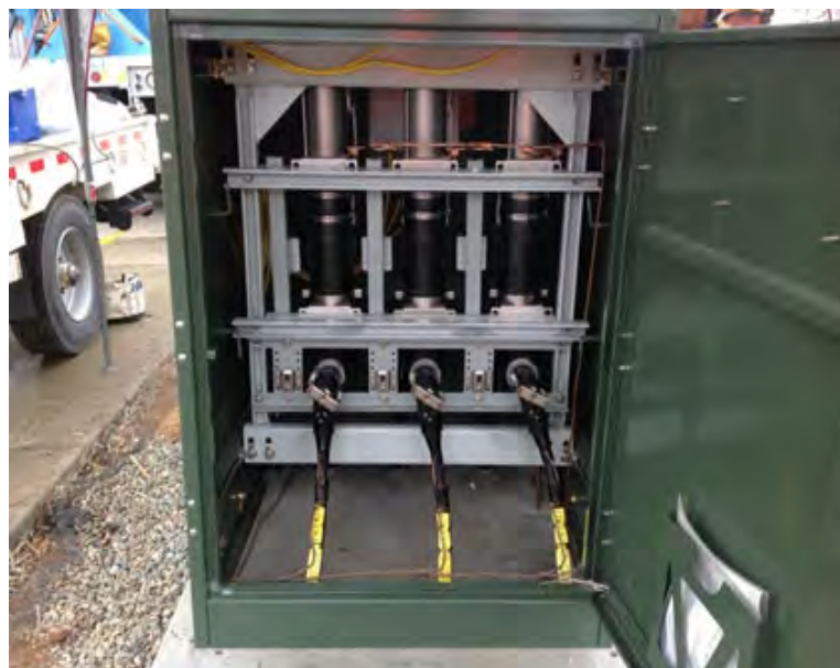
Figure 7 PMI-4R Single Phase Vacuum Fault Interrupter – Load Side (replacement construction shown)
