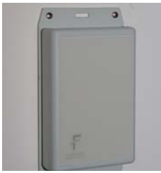
DART Sensor Located outside diffuser for ceilings with Asbestos issues
