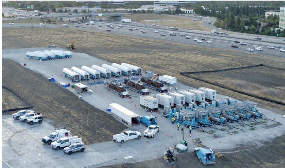
Figure 25 – A Large-scale LNG injection Site in Dublin, CA Supporting a Planned Gas Outage
