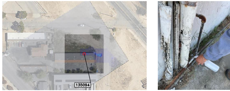
Figure 72 – (L-R) Shows a leak indication from the aerial photography report – Aligns with the actual leak location
