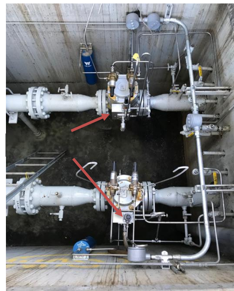
Figure 44 – Photo Pointing to Slam Shut Installations
