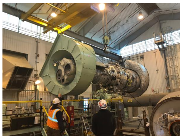
Figure 18 – Delevan Compressor Station Turbine Exchange
