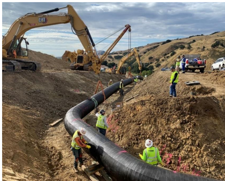
Figure 68 – Field installation of the advanced distributed fiber optic sensor monitoring systems on L-300B at a Calaveras Fault-crossing site in Gilroy.
