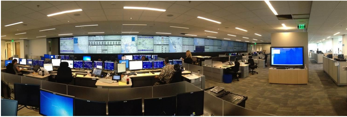
Figure 39 – PG&E’s Gas Control Center Features a 90 Foot-Long Video Wall With Current Operational Information to Augment The Gas SCADA System (Photo Captured Pre COVID-19)
