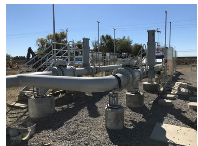
Figure 16 – M&C Complex Station-Above Ground
