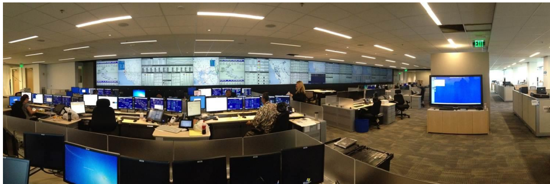
Figure 43 – PG&E's Gas Control Center Features a 90 Foot-Long Video Wall With Current Operational Information to Augment The Gas SCADA System
