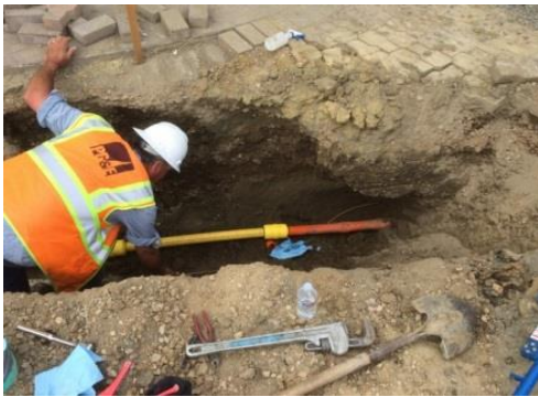
Figure 53 – Supported 276 811 Dig-In Reduction and safety-related activities in collaboration with the Damage Prevention team to improve safety within PG&E’s communities and reduce the incidents of third party dig-ins.
