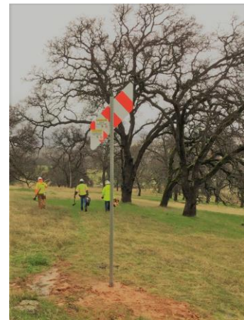
Figure 25 – Crew After Completion of the Installation of a New Pipeline Crossing Marker
