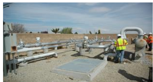
Figure 14– M&C Simple Station-Above Ground
