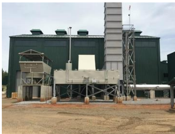
Figure 12 – PG&E’s Burney Compressor Station
