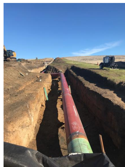
Figure 13 – L-131 Newly Installed Transmission Pipe
