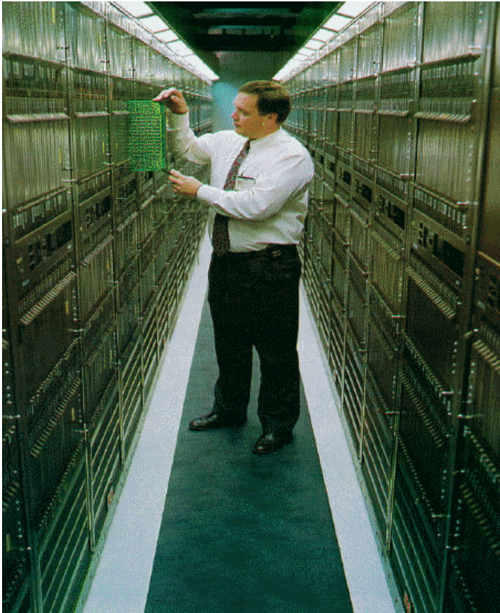
Long-distance calls from around the world are handled in Sprint's digital switching centers.
