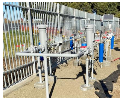
Figure 21 – Large Volume Customer Facility
