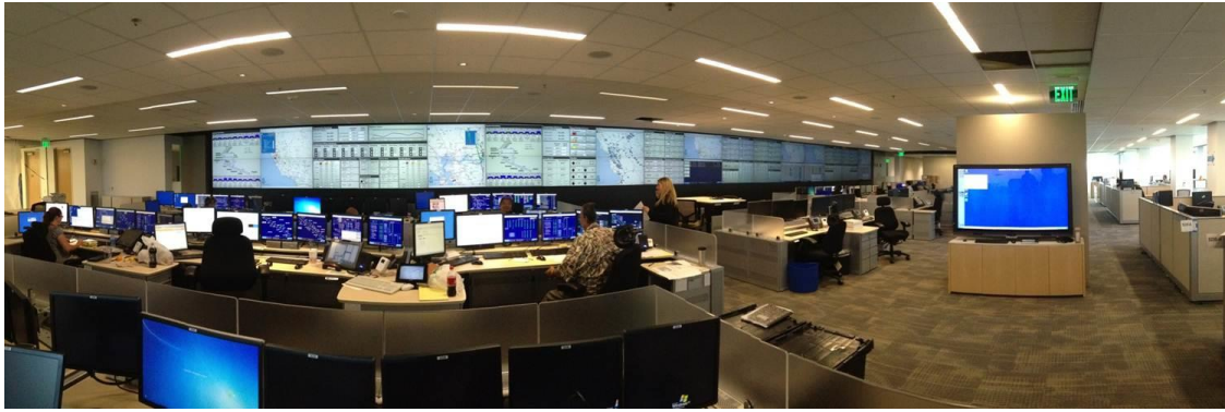
Figure 50 – PG&E’s Gas Control Center Features a 90 Foot-Long Video Wall with Current Operational Information to Augment the Gas SCADA System
