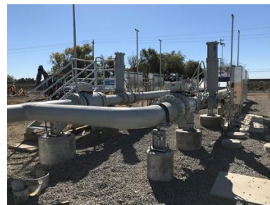
Figure 20 – M&C Complex Station Above Ground
