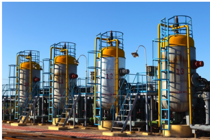
Figure 7 Industrial Pressure Swing Adsorption Plant (AIChE, 2014)
