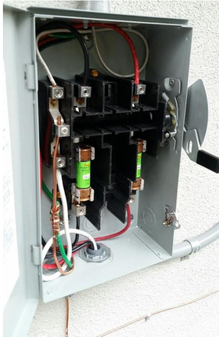
Figure 6. LFNC Conduit and Wires Connected in PG&E Approved Fused Disconnect Switch
