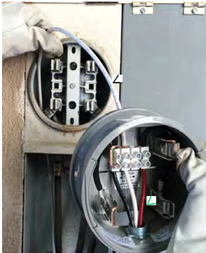
Figure 5 Extend Insulated Wires Past the LFNC Conduit
