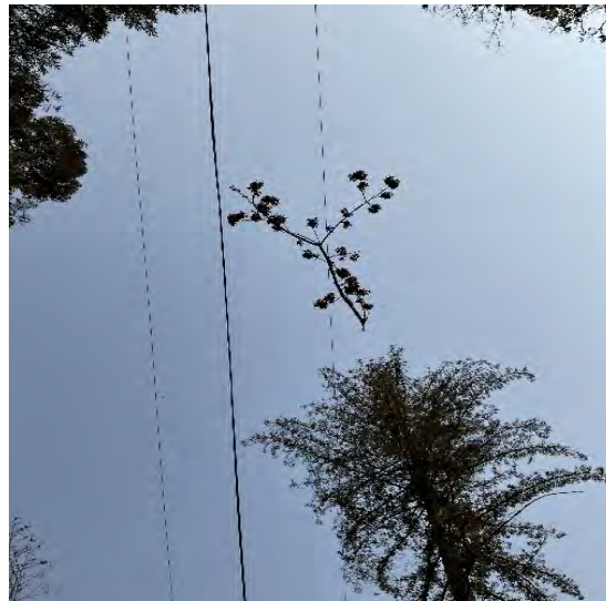
Figure 18: Vegetation-Hazard in Napa County – Tree Branch on Line
