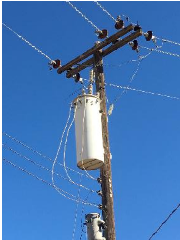
Figure 13: Wind Damage in Kern County – Broken Cutouts
