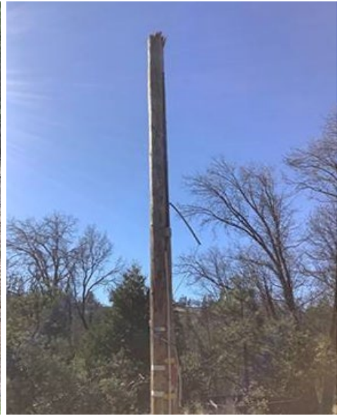
Figure 16: Vegetation-Caused Damage in Madera County – Tree Fell Breaking Pole and Conductor
