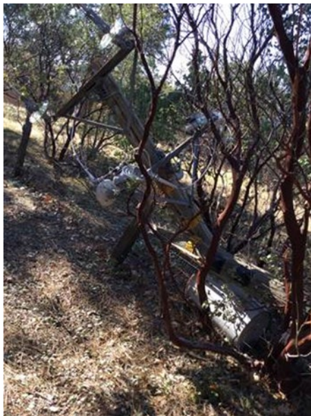
Figure 17: Wind-Caused Damage in Mariposa County – Pole Brought Down at Base, Line Down
