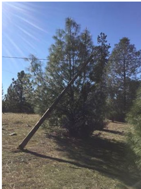
Figure 18: Vegetation-Caused Damage in Mariposa County – Tree Fell Through Service Breaking Pole
