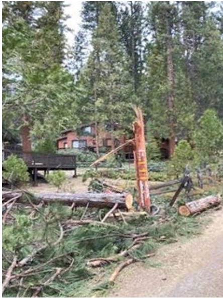
Figure 14: Vegetation-Caused Damage in Mariposa County – Tree Failed into Lines and Broke Pole
