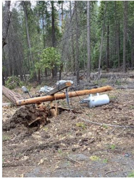
Figure 15: Vegetation-Caused Damage in Mariposa County – Tree Took Down Lines and Broke Pole
