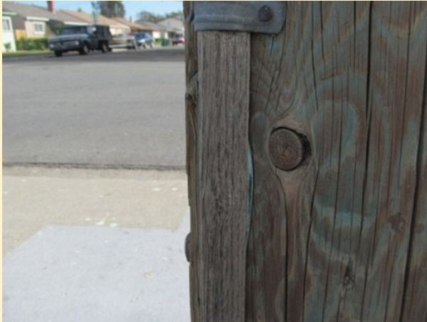
Before: Copper Wire sticking out from under the wood molding
